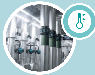
HVAC & Swimming Pools
